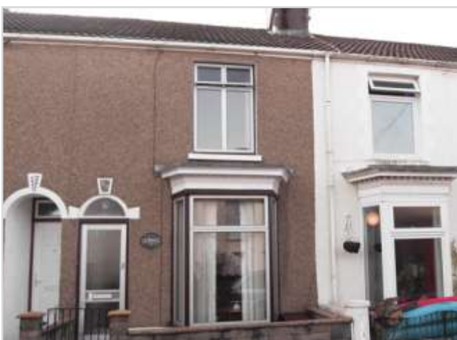
Changes to wall finishes, door and window openings and frames remove the heritage character and the rhythm of the terrace
